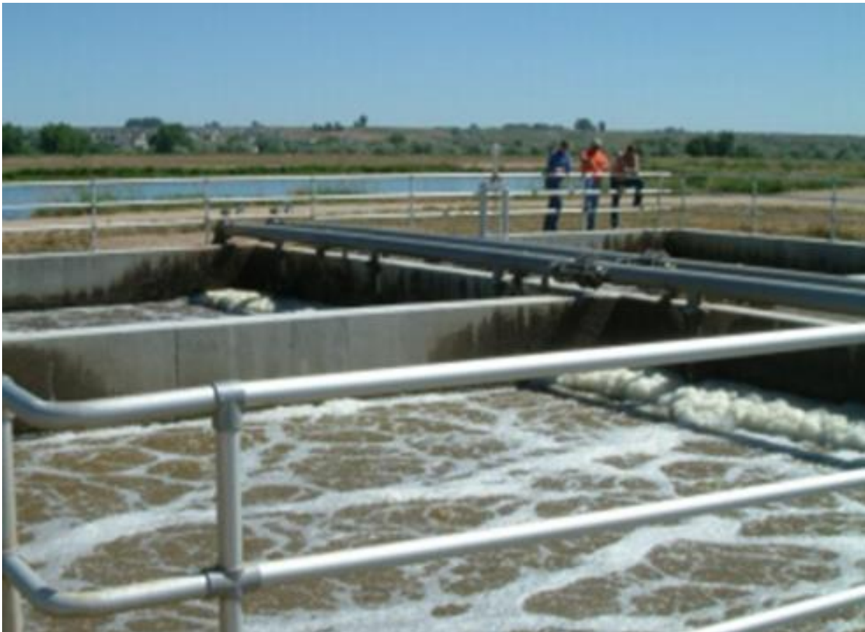
Figure 26: LagoonGuard MBBR operating with a lagoon in the background
