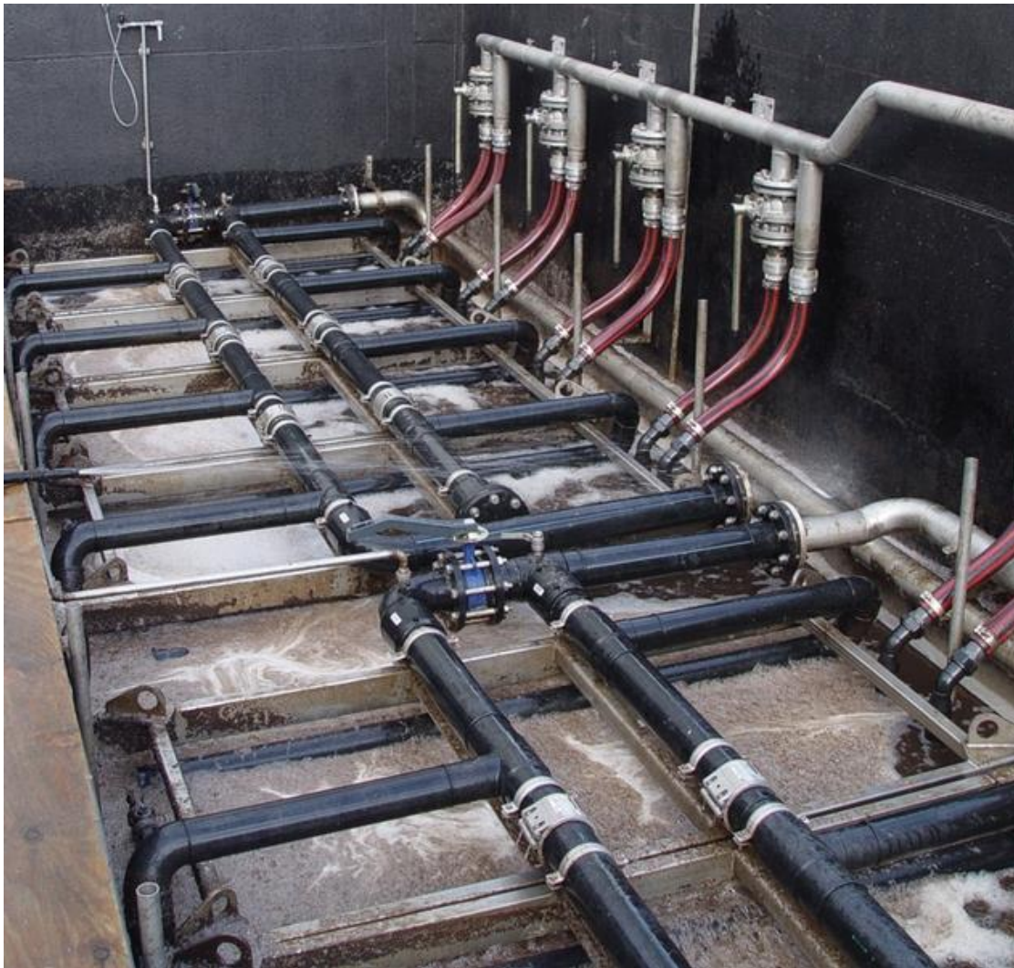
Figure 35: Aqua Aerobic MBR system
