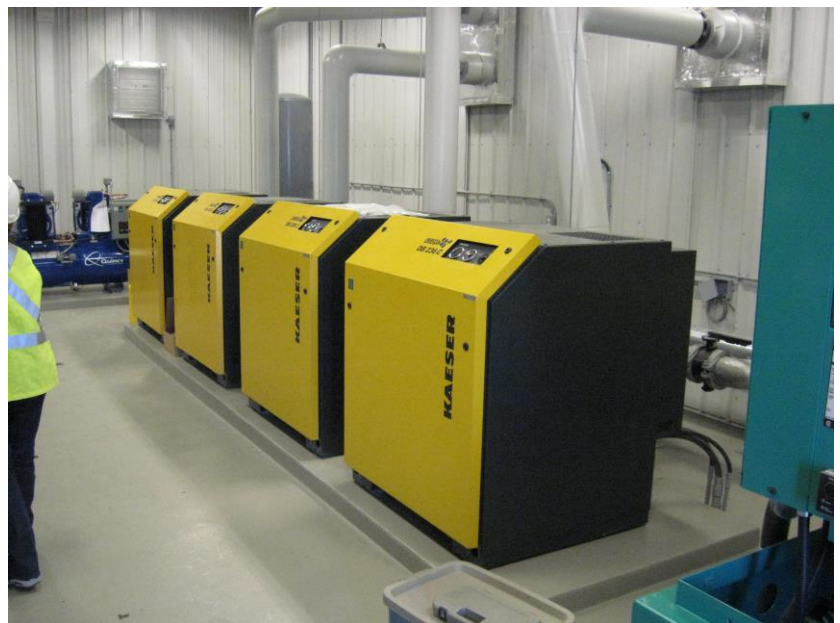
Figure 24: Example of the blowers required to operate the SAGR system [24]
