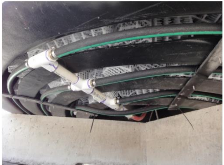
Figure 12: Bottom of Bio-Dome showing concrete base, air manifold and packing [17]
