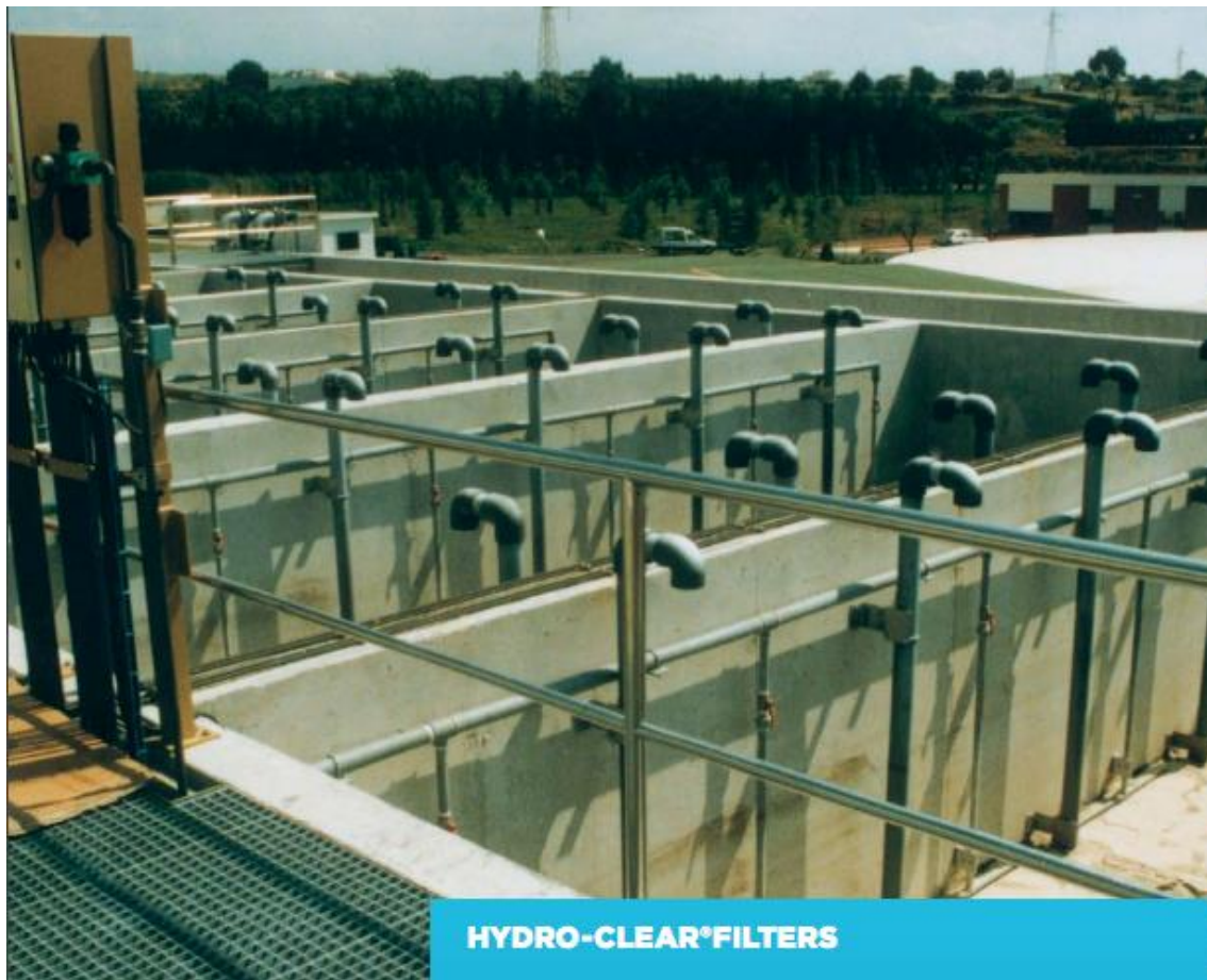
Figure 31: Hydro-Clear sand filtration unit
