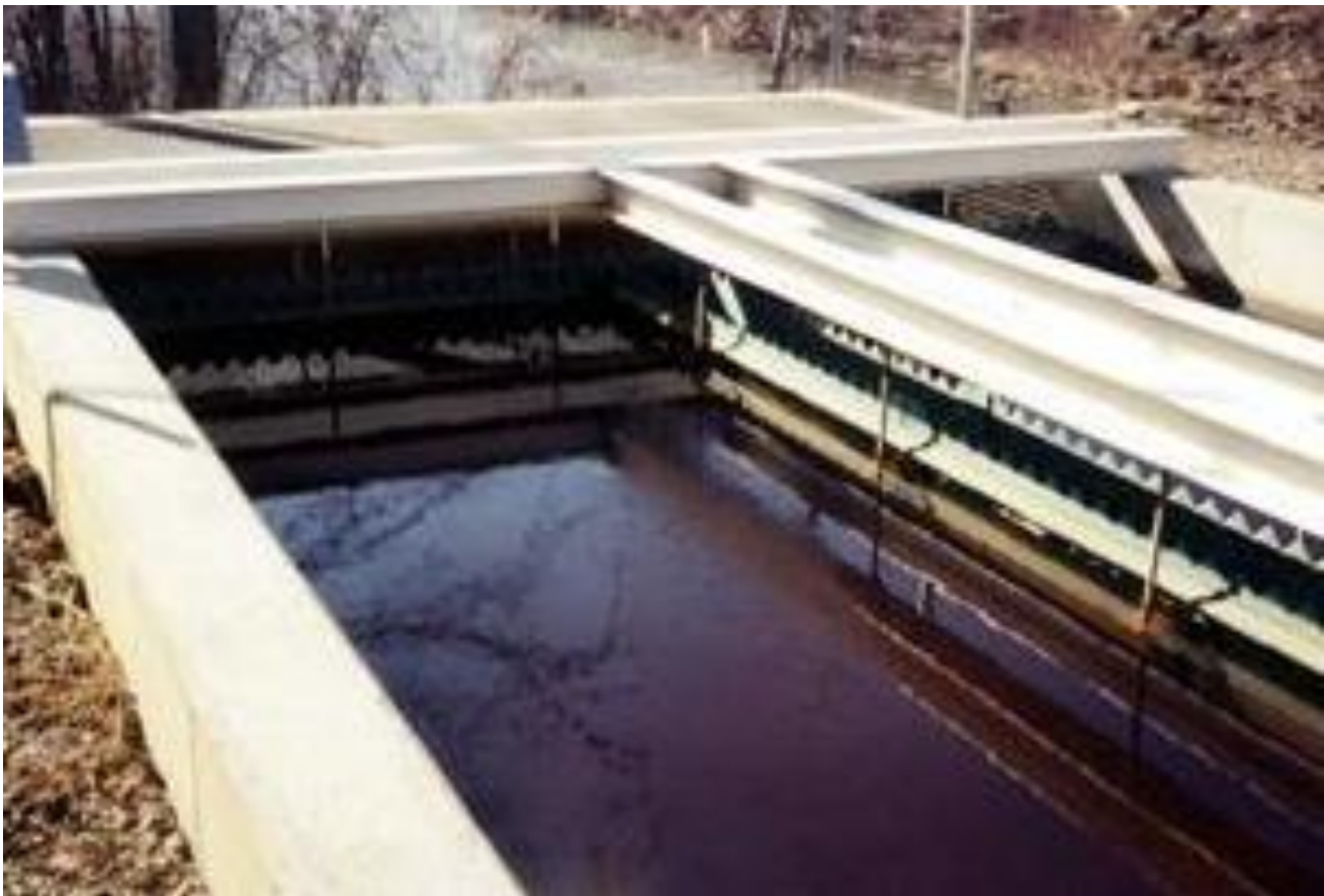
Figure 40: AQUA-4 treatment system installed at a wastewater treatment plant
